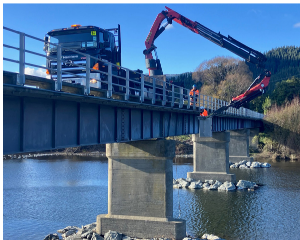
Investigation work was undertaken in May on Dalton's Bridge to inform design for the abutment repairs
