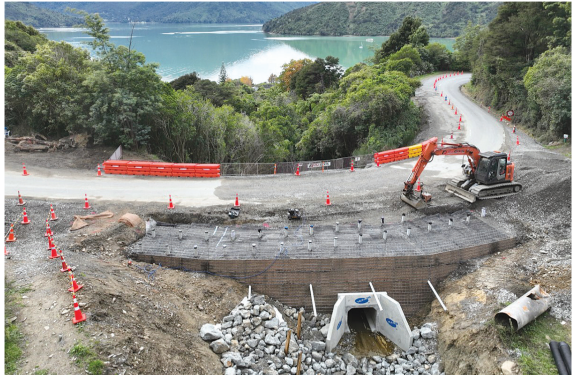
More repairs like this one at Moenui, Queen Charlotte Drive are signalled with Council's decision to fund the Sounds roads repairs
