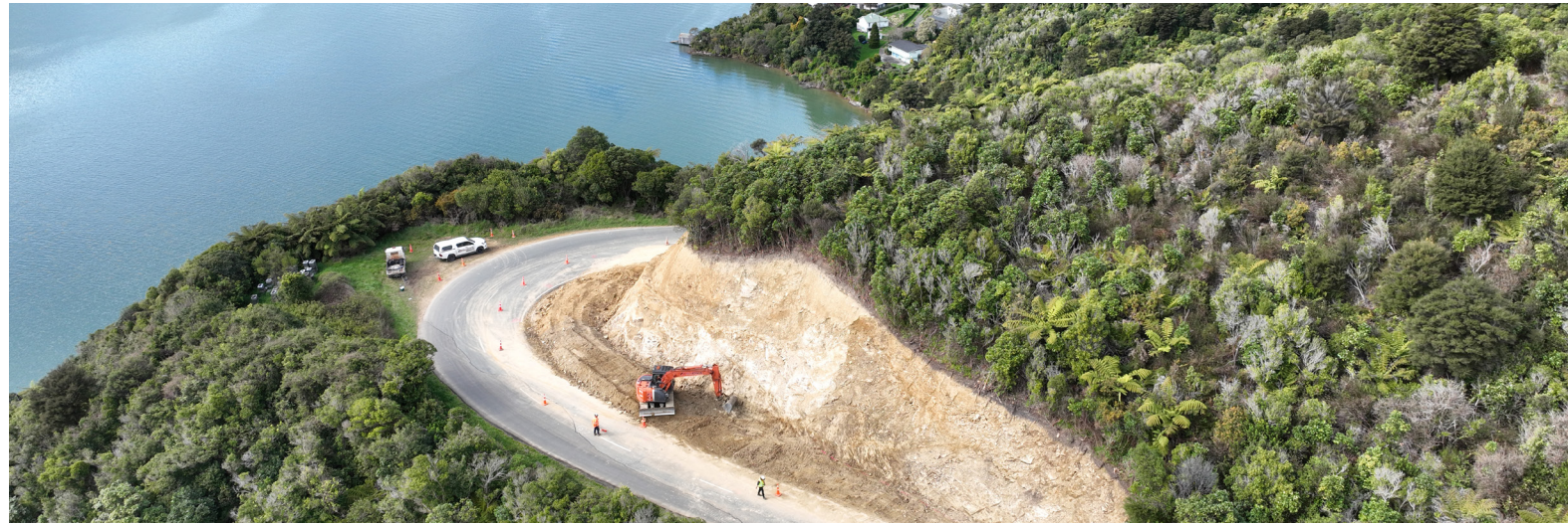
Recovery work in the Sounds can pick up speed now that NZTA have confirmed funding for the repair stage of phase three of the Sounds recovery roading programme
