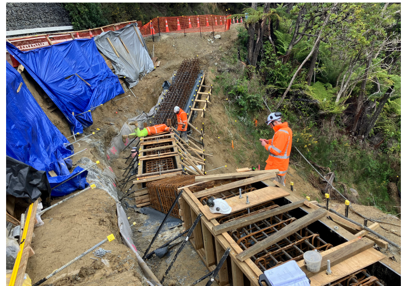
📷 Ongoing Sounds recovery works such as the Torea Wall near Portage Bay form part of a very complex Long Term Plan, adopted by Council
