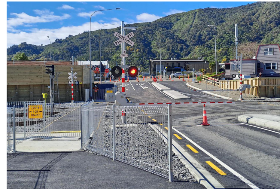
Barrier arms and signals, and a new pedestrian safety feature, a 'maze', on the level crossing have been installed at Dublin Street
