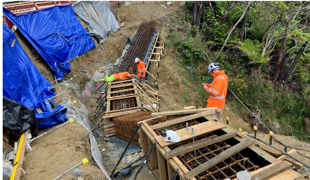
Ongoing Sounds recovery works such as the Torea Wall (pictured) near Portage Bay form part of a very complex Long Term Plan, adopted by Council earlier this week
