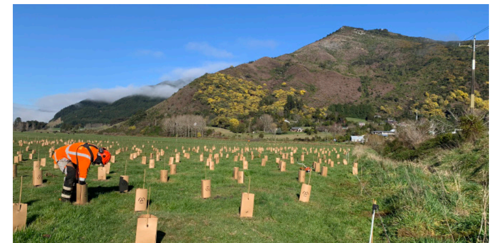
J&S Mears Contracting is planting natives for the project, using plant guards that are biodegradable and give seedlings the best chance of survival
