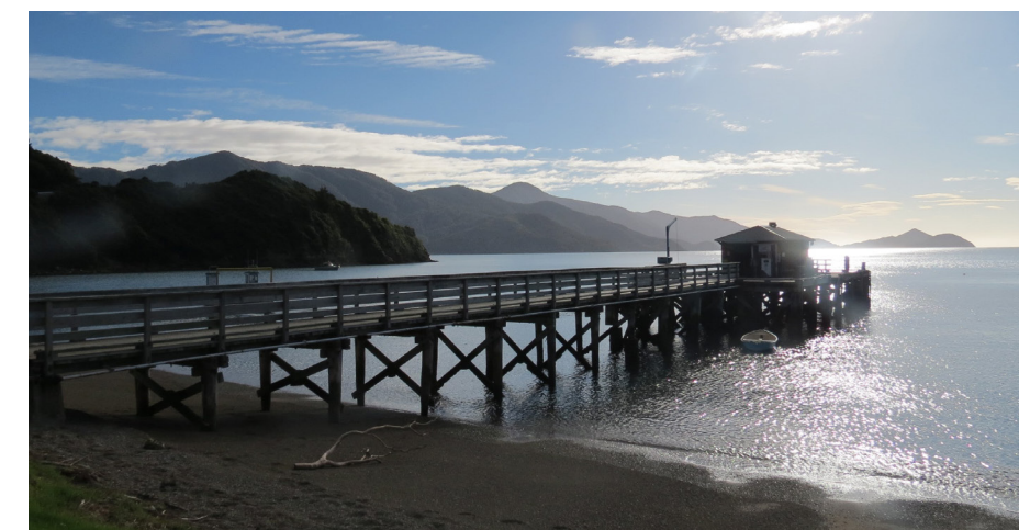
The Elmslie Bay jetty is at the end of its life and needs replacement
