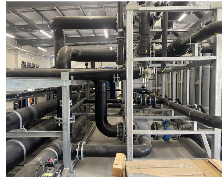
Renwick's new water treatment plant which became operational in June already supplies treated chlorinated water to all properties in urban Renwick
