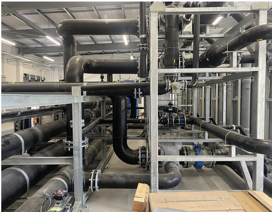
Renwick's new water treatment plant which became operational in June already supplies treated chlorinated water to all properties in urban Renwick
