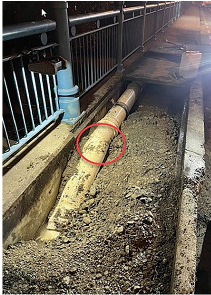
The damaged water main on the Sinclair Street bridge
