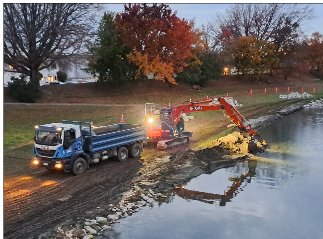
📷 A digger works on removing sediment from the Taylor River in front of the ASB Theatre
