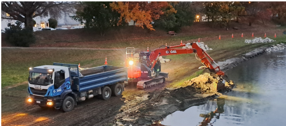
A digger works on removing sediment from the Taylor River in front of the ASB Theatre
