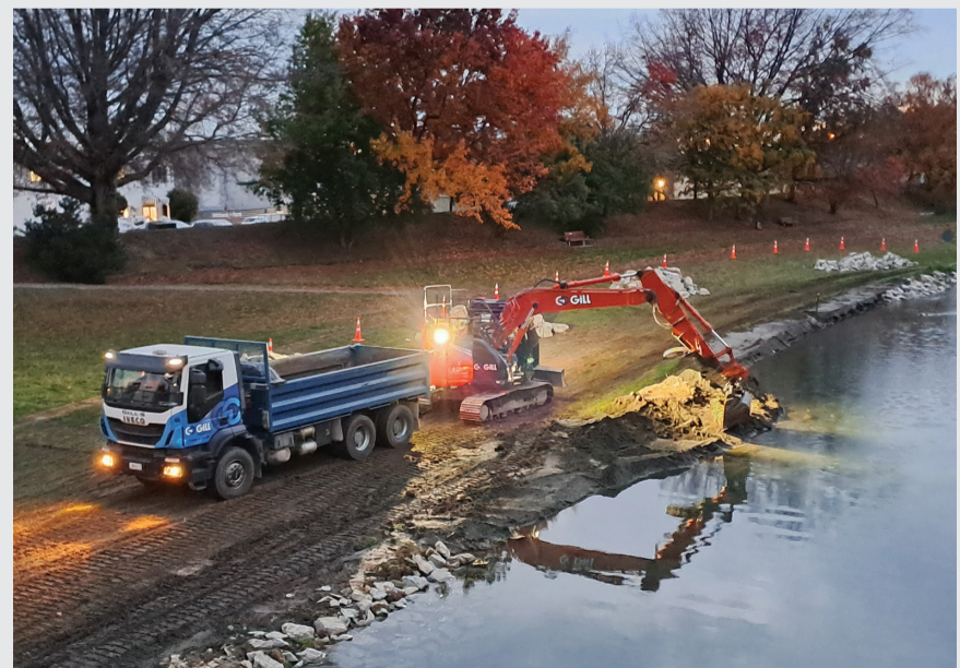
A digger works on removing sediment from the Taylor River in front of the ASB Theatre
