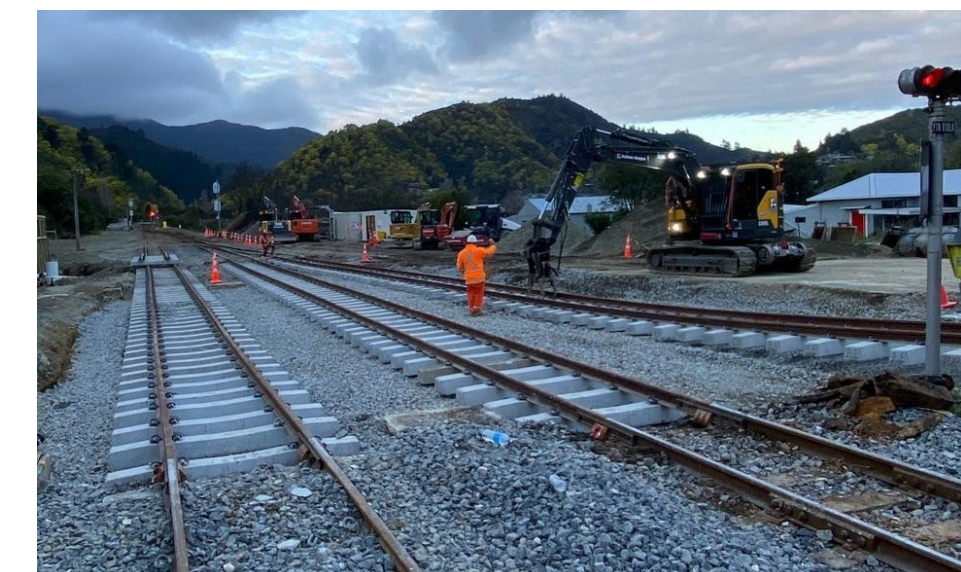
KiwiRail is focused on getting the Dublin Street level crossing barrier arms and signals reinstalled ready for reopening at the end of this month
