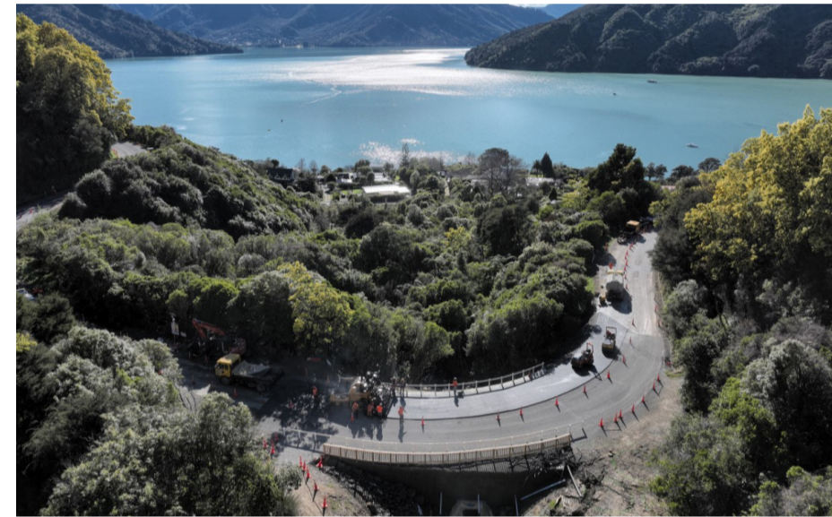
A site near Moenui Road is one of two complex repairs completed on Queen Charlotte Drive
