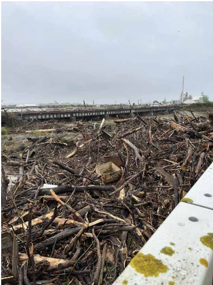
Figure 8.12 Debris at Waitangi Railway Bridge and road bridges immediately downstream of Awatoto stopbank breach 187
