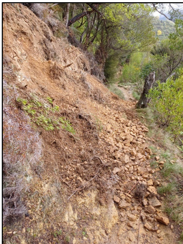
Tirohanga Track slip
