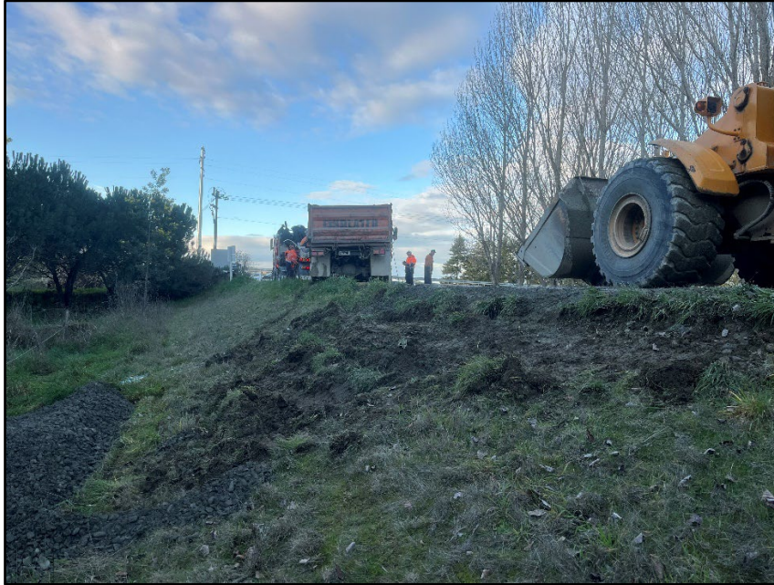
Figure 4 - Damaged river face of main stopbank
