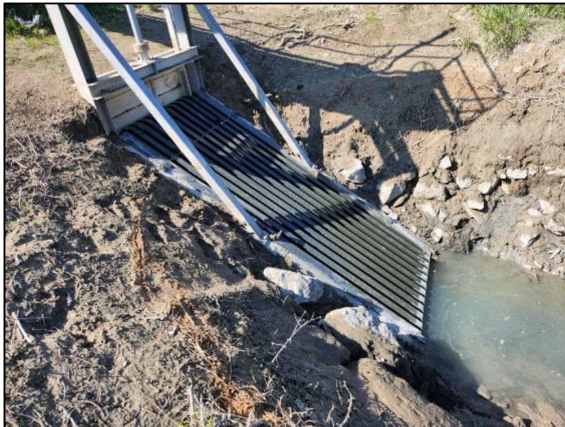
Figure 9 - Debris screen added
