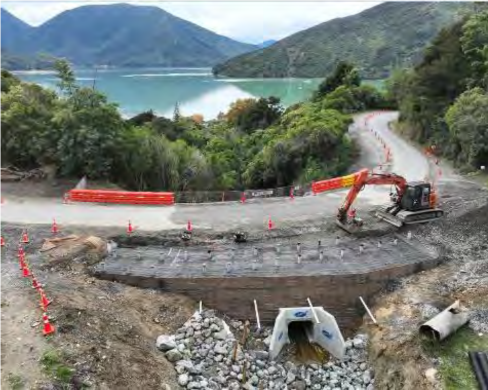
MSE head wall built up at the Moenui box culvert installation site – 24 May 2024
