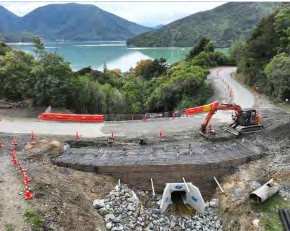
MSE head wall built up at the Moenui box culvert installation site – 24 May 2024
