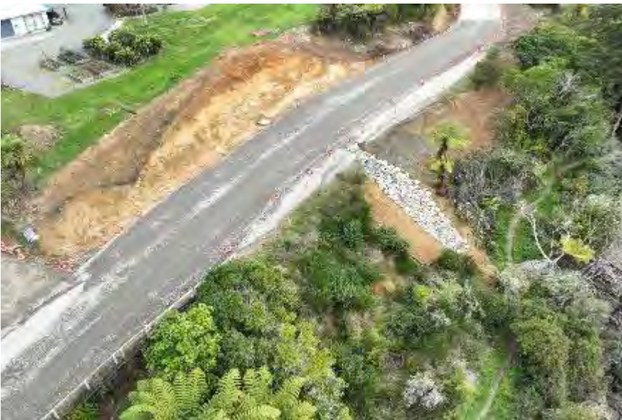
Retreat and new culvert installation on Queen Charlotte Drive, near Tepuia Heights – 23 May 2024
