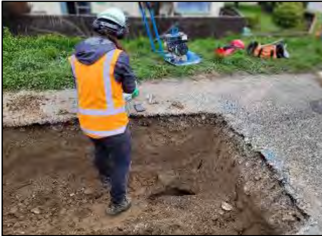
Figure 8 - cracking and voids within stopbank
