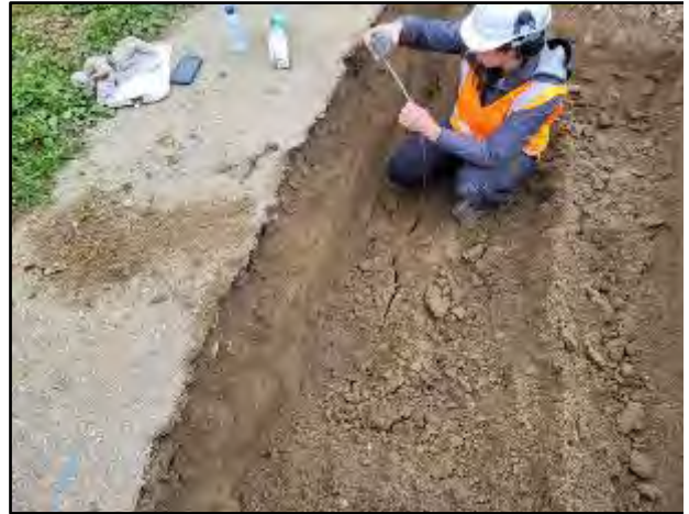
Figure 9 - recording cracks within stopbank
