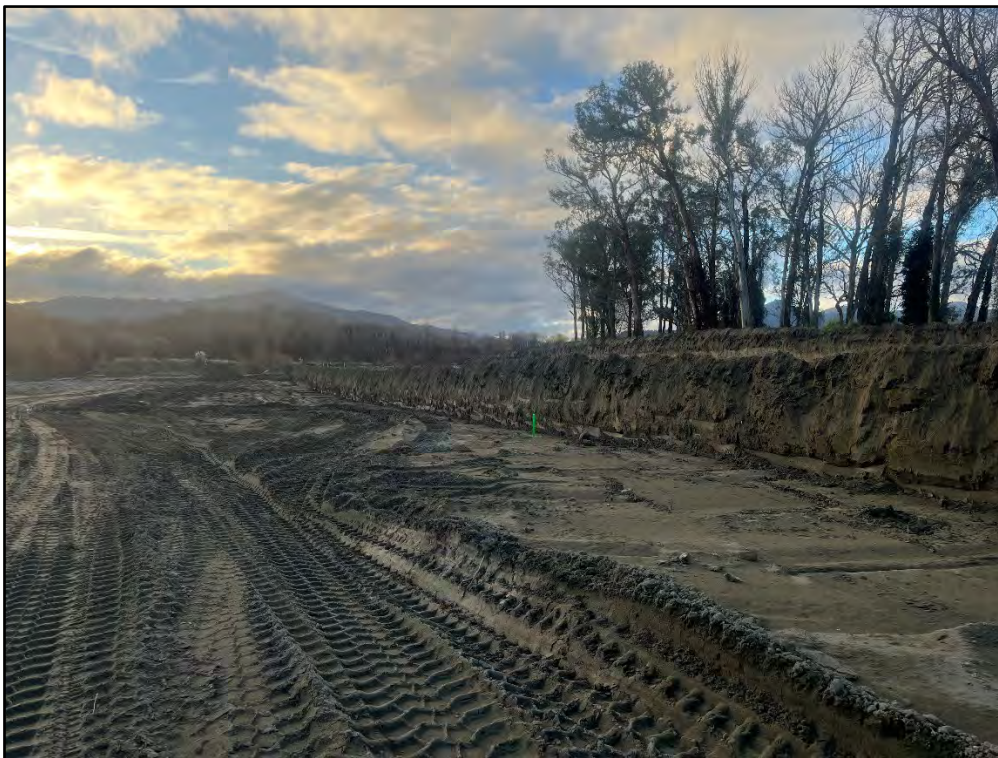
8 - green pegs for contractor to set the toe of the new edge
