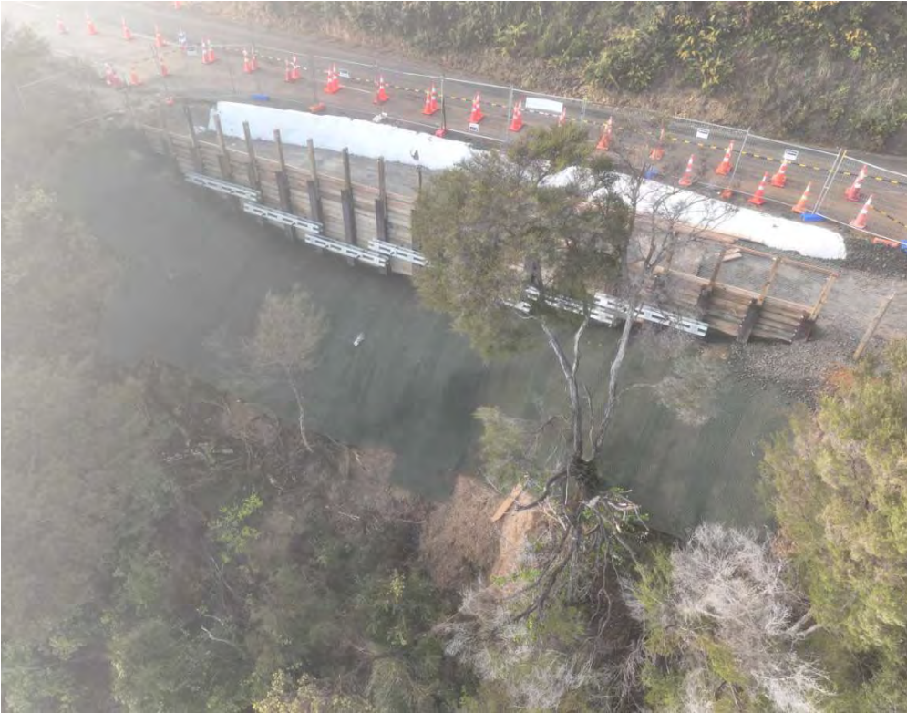
Second wall at Aussie Bay, fill and compaction underway and geo-mesh in place – 21 June 2024
