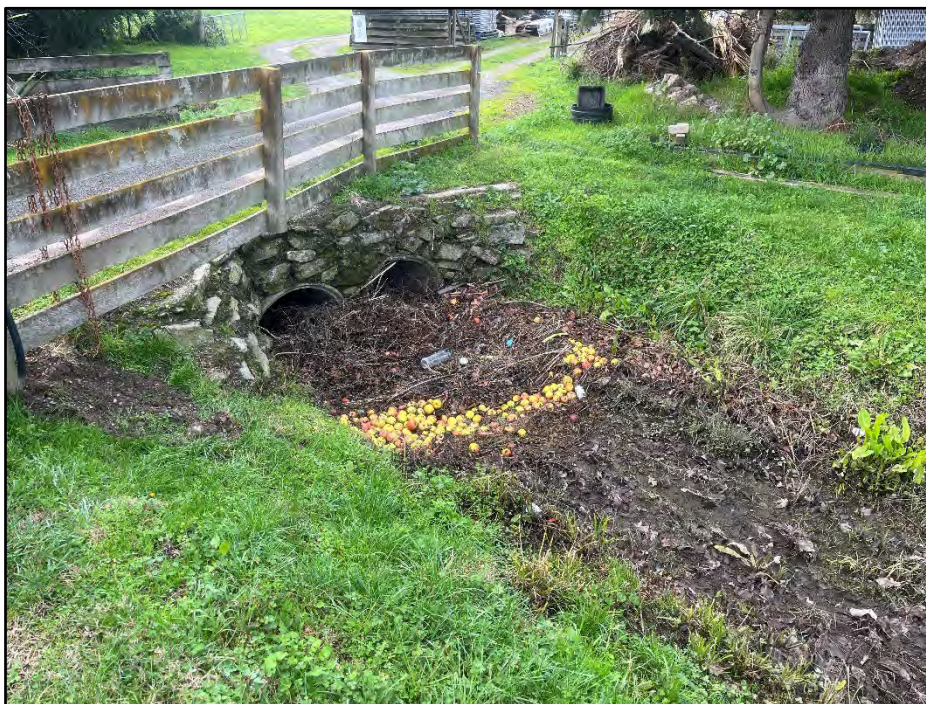
11 - blocked twin culvert in School Creek
