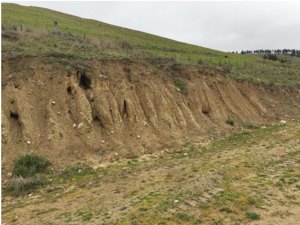
Photo 2: Tunnel gully and rilling erosion in north facing cut face on the southern flanks of 15 th Valley
