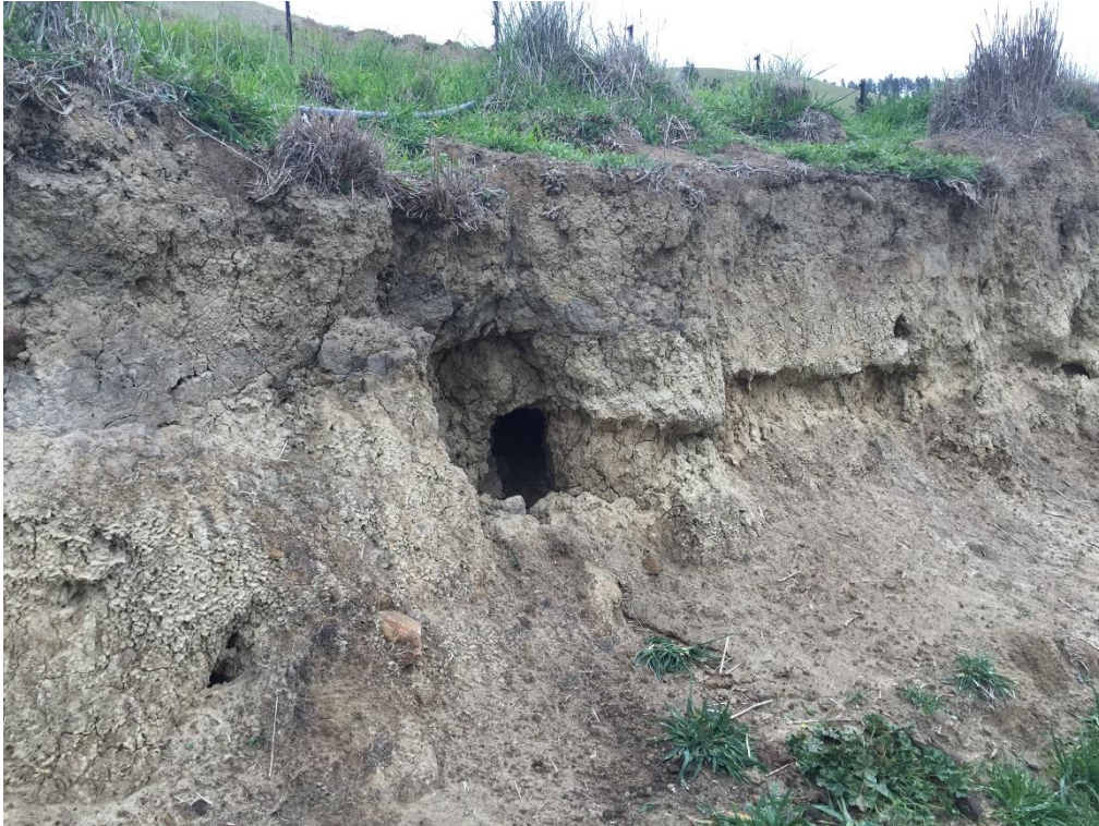
Photo 3: Tunnel gully erosion on north facing foot slope (southern valley flank) of 15th Valley
