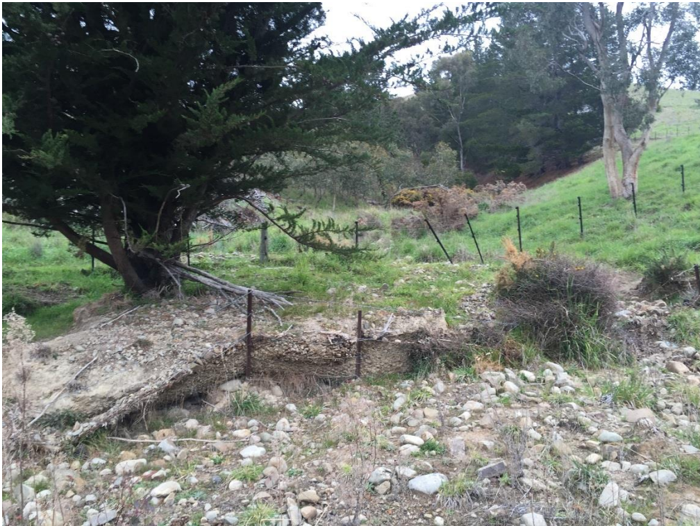
Photo 4: Shallow debris flow from secondary valley caught by fence within drainage channel
