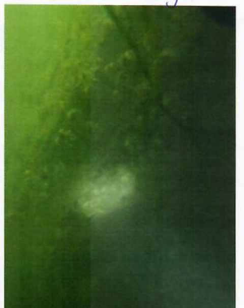
Marine growth on inside of pipe line.
