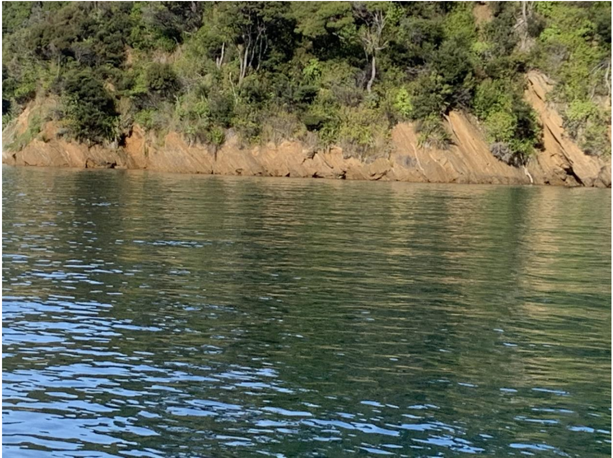
Photo 3: Rock slope along northern end of property towards dilapidated boatshed and fixed jetty
