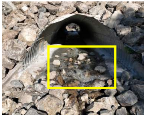
1.5m pipe diameter – Awatere
